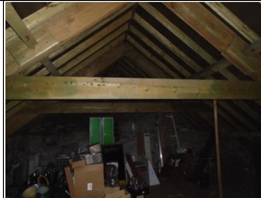
Photo 30. Lodway Farm Building LF7 – the interior of the barn shows the new roof structure. Date: October 2018
