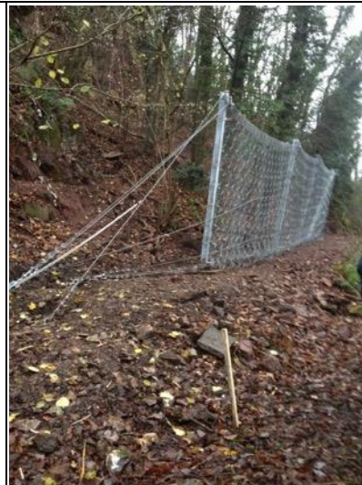
Photo 8. Portbury Fright Line (Rock Fall Prevention Fence) Date: December 2015
